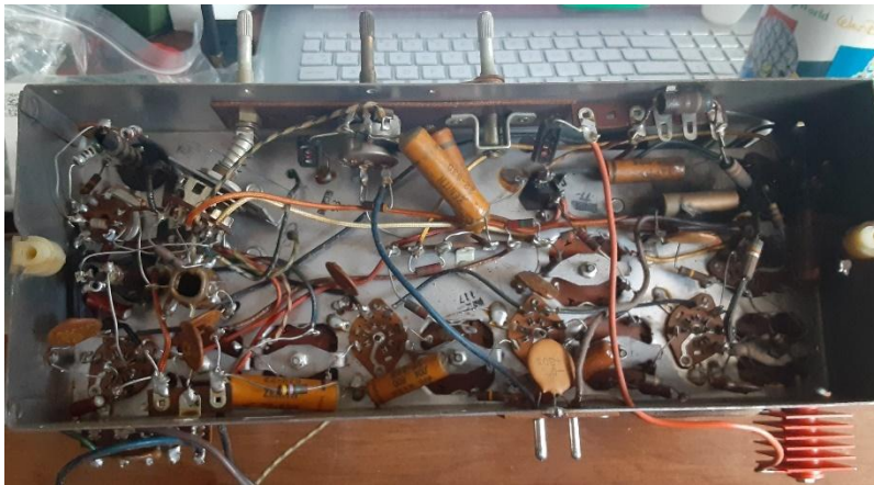
Figure 2 - Under-chassis view before repairs
