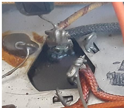
Figure 12 - Electrolyte leaking from filter capacitor
