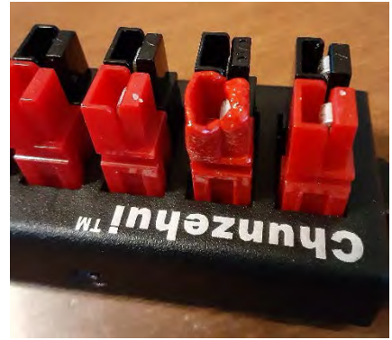
Figure 4 - Melted block port
